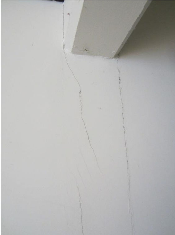
Foto C1: Geringe scheurvorming begane grond
